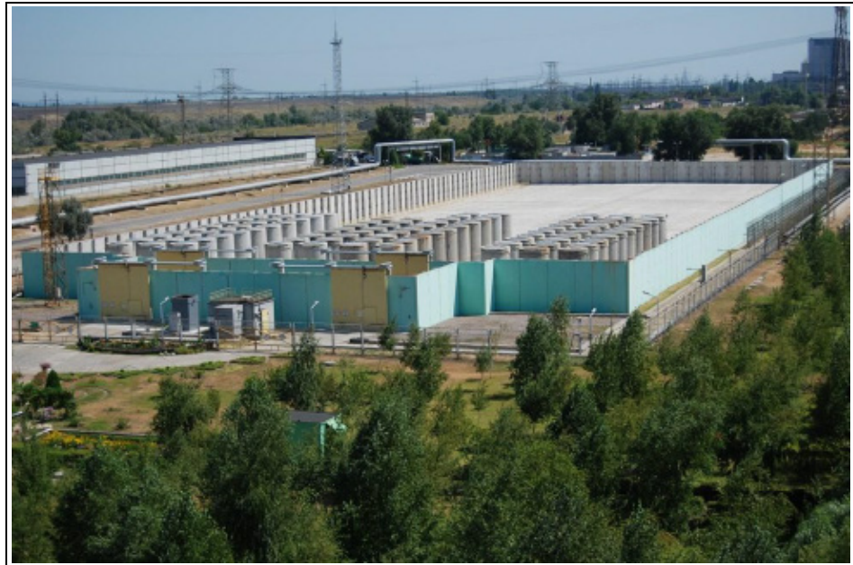
Figure 3: ZNPP dry interim storage for spent fuel (DSFSF)
