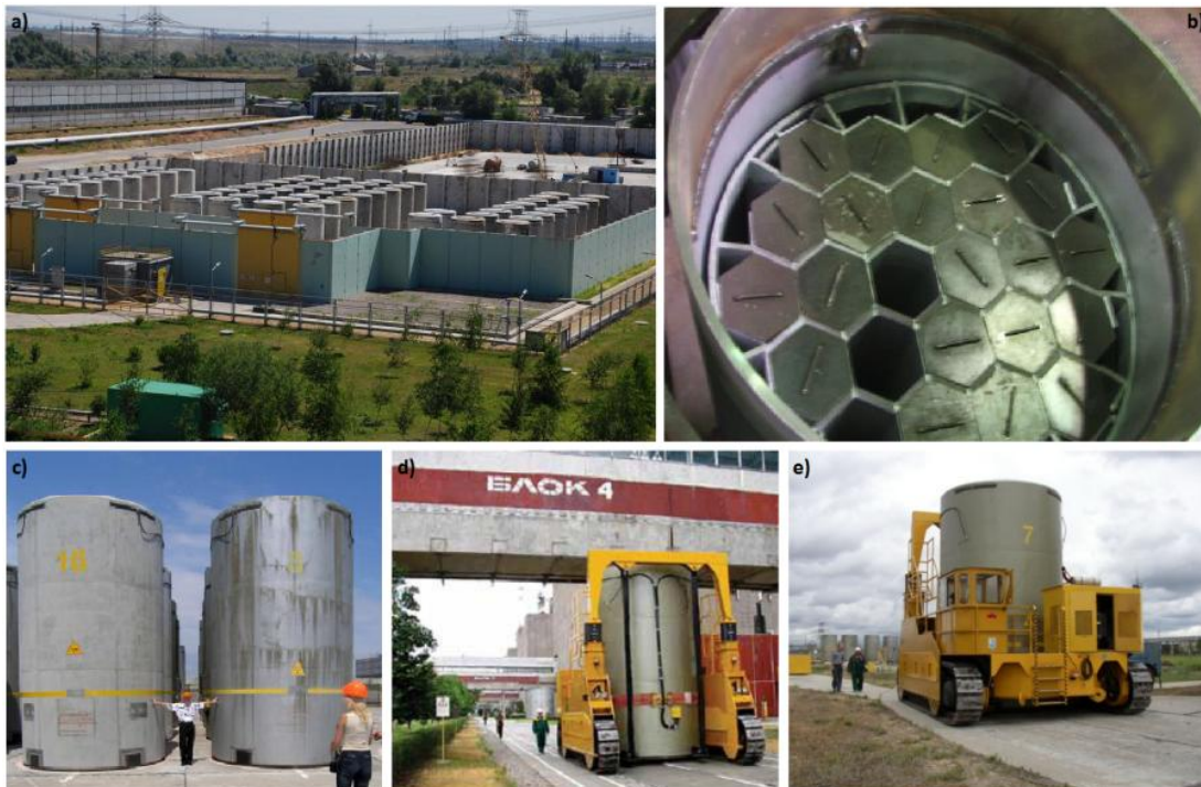
Fig. 16 Interim storage facility at the Zaporizhzhya NPP (Energoatom, 2010)
