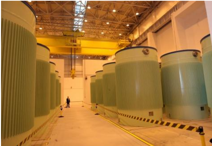
Fig. 18 CONSTOR type containers in the interim storage facility Kozloduy (IAE, 2005)
