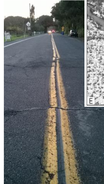
2014 West Napa quake surface faulting : tar road offset measured 0.4 m in Dec. 2014
