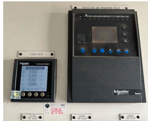
The energy meter (Schneider PM5560 0.2S)
