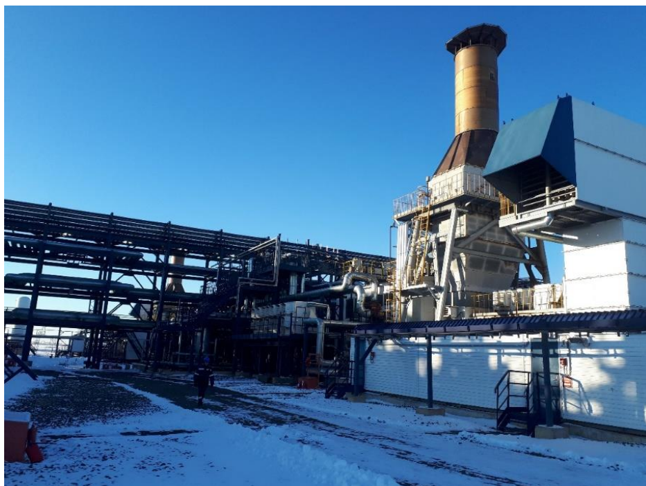
Figure B: New compressor unit
