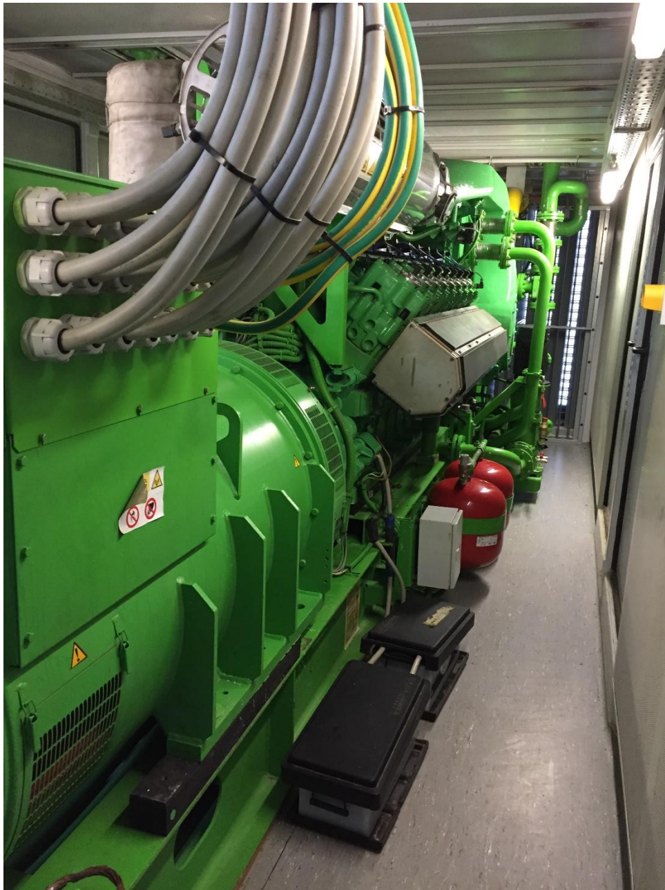
Image 4: Gas engine and electrical generator set group 2
