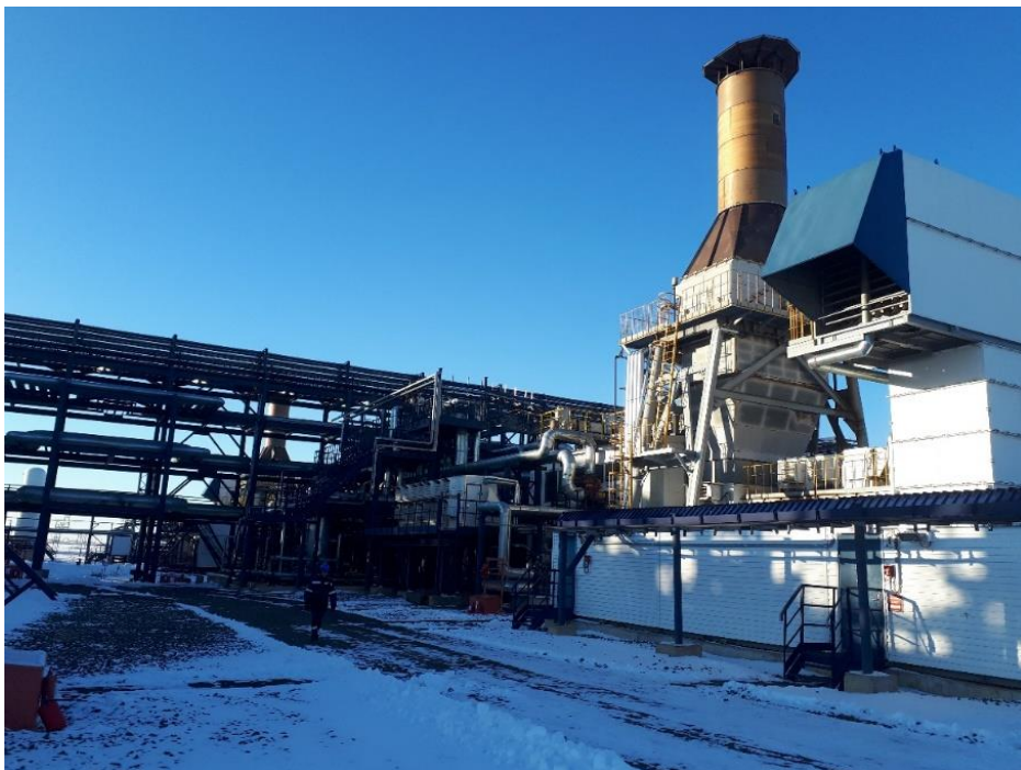
Figure B: New compressor unit
