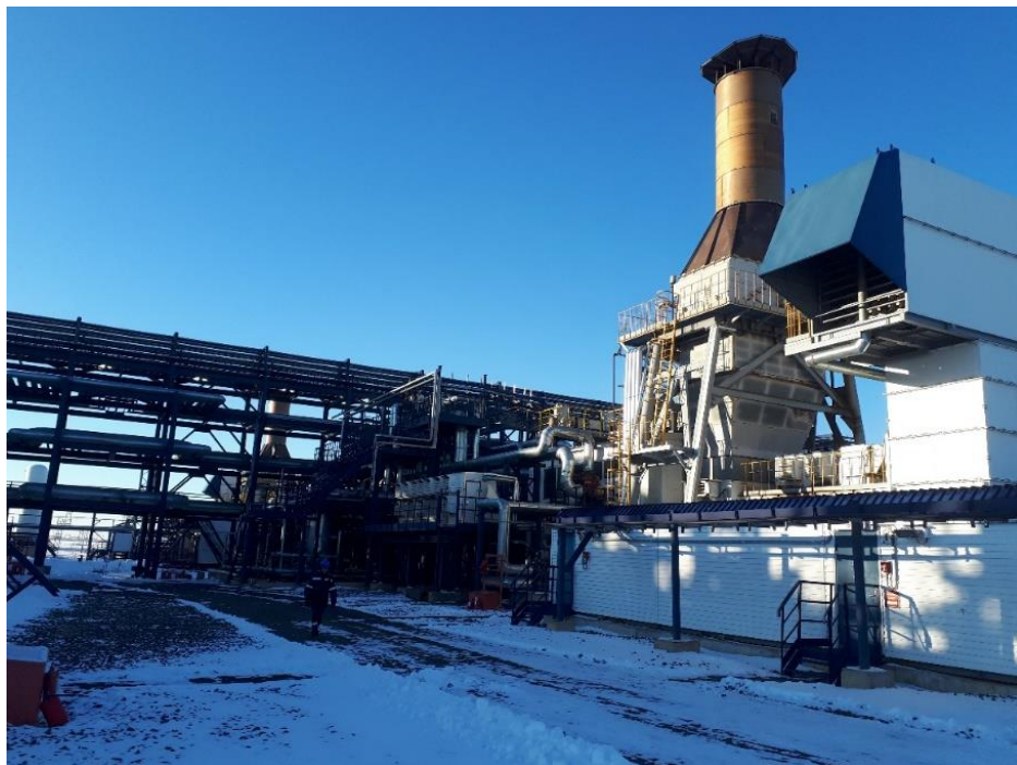
Figure B: New compressor unit
