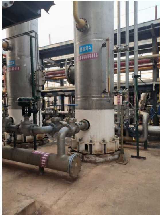
Image 2: The skid of desulphurization
