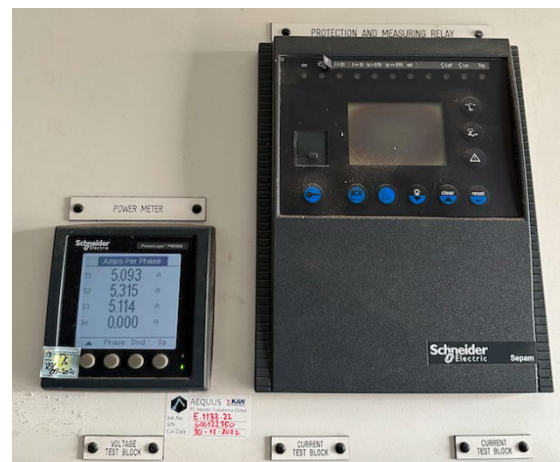
The energy meter (Schneider PM5560 0.2S)
