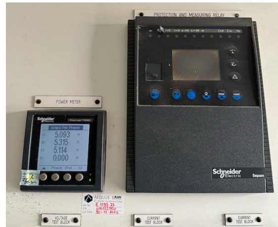
The energy meter (Schneider PM5560 0.2S)
