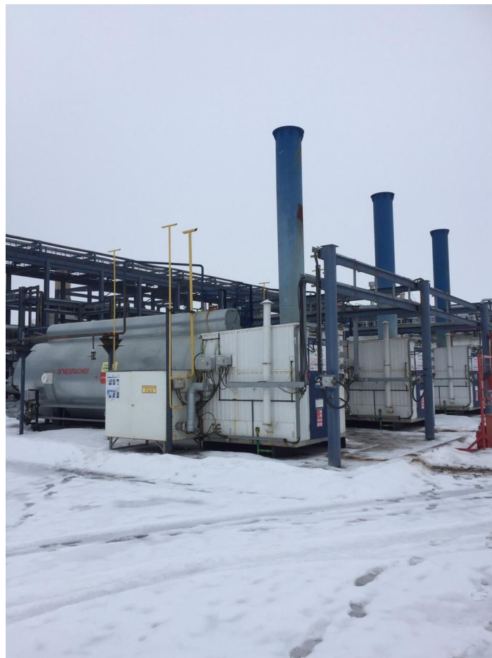
Figure D: Oil and gas processing facilities
