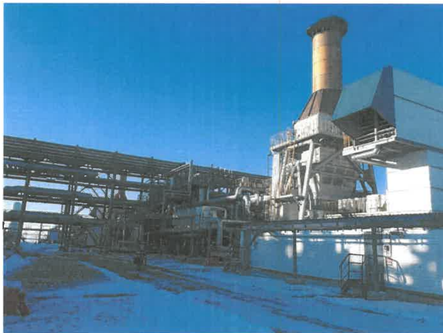
Figure B: New compressor unit
