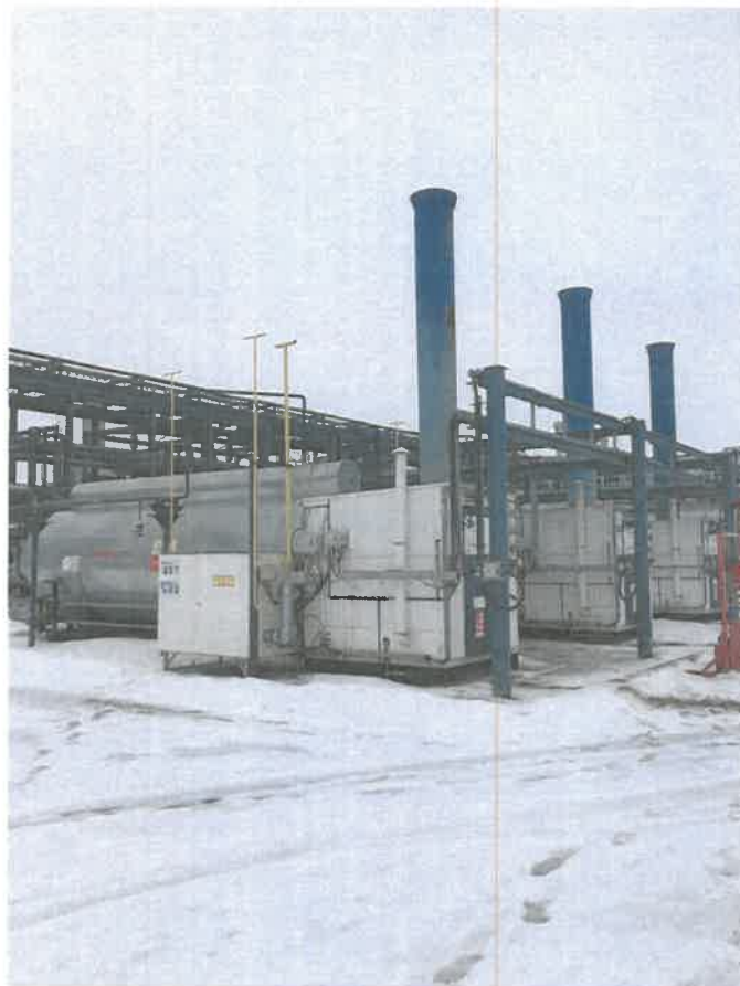
Figure D: Oil and gas processing facilities
